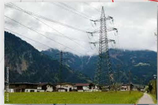
High voltage lines
